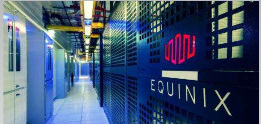
Equinix Data Center
